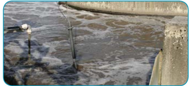
In the aeration: calibration free FDO 700 IQ F for dissolved oxygen
